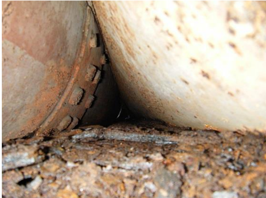
Plate 2 - Slight or insignificant corrosion to upper segments within closed bottom section
