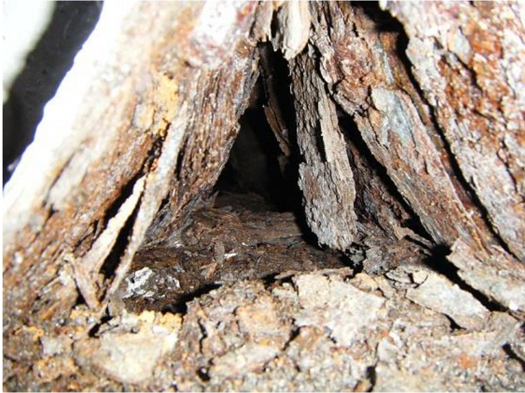
Plate 1 – Very significant corrosion within closed bottom section
